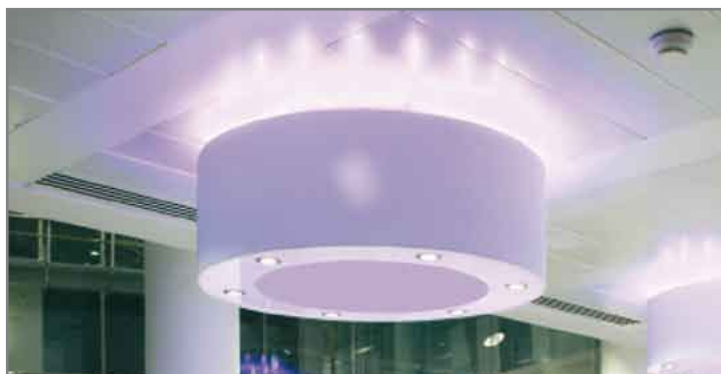
Figure 5: The fixture is equipped with warm white LED light engines for task lighting and blue LEDs for ceiling accent lighting
