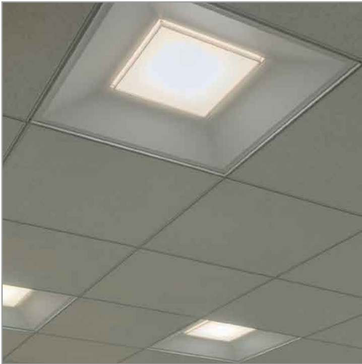
Figure 3: LR24 luminaries, such as the ones shown here, are being used in place of fluorescent fixtures in the Pentagon
