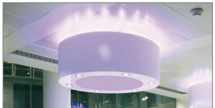
Figure 5: The fixture is equipped with warm white LED light engines for task lighting and blue LEDs for ceiling accent lighting
