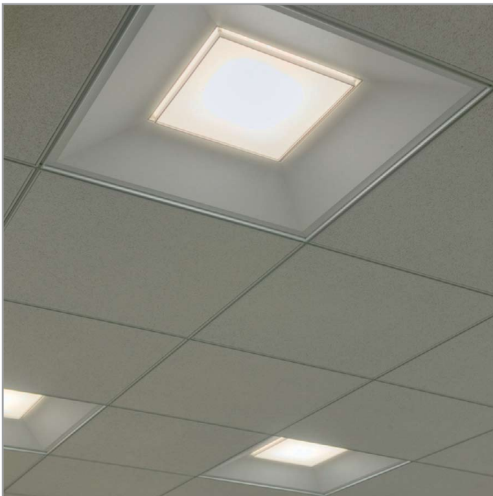
Figure 3: LR24 luminaries, such as the ones shown here, are being used in place of fluorescent fixtures in the Pentagon
