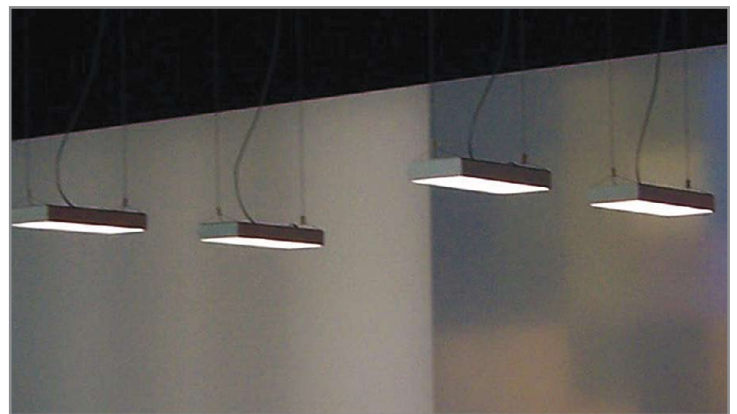
Figure 7: Pendant LED luminaires for office applications. Light is emitted by 11 high power LEDs and directed towards the work space by a microstructured optical cover. Glare reduction is also performed by the microstructure.
