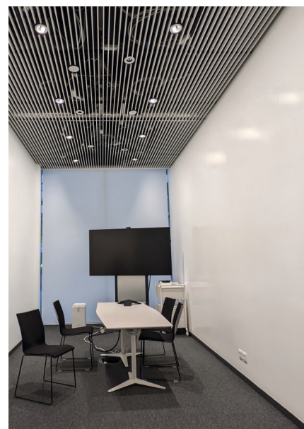
Meeting room with LMT Leuchten + Metall Technik GmbH "NAU" RJR wallwash downlight with Optisolis in 3000K. Photo credit: LMT GmbH.
