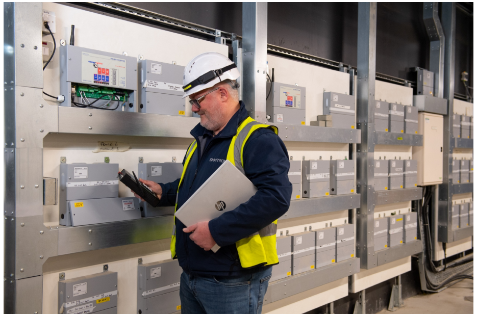
Control Room with Simmtronic Equipment. Image credit: Simmtronic / Jon Parker Lee Photography.
